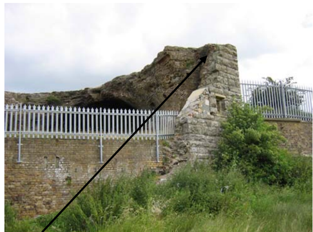
2 Site of fall (fencing was put in afterwards)
